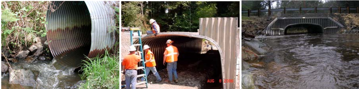
Yonkers Creek Migration Barrier Removal Project (Del Norte County 2006) Left - Before, Middle - During, Right - After
