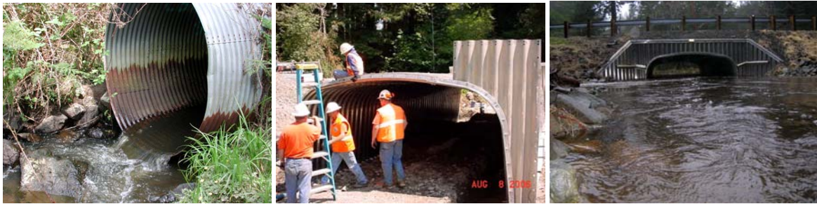
Yonkers Creek Migration Barrier Removal Project (Del Norte County) Left - Before, Middle - During, Right - After
