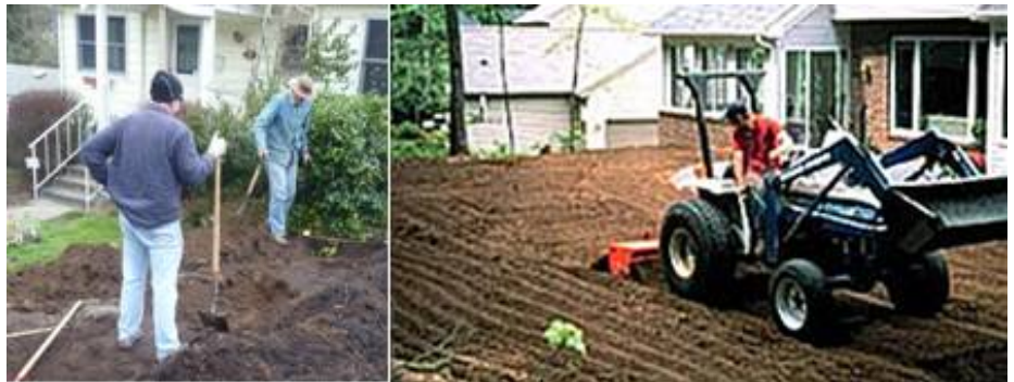
Figures 4 & 6. A range of construction equipment (tiller, cat mounted ripper, tractor-mounted disc, etc) or simply shovels and rakes may be used depending on the extent of the area to be amended.
