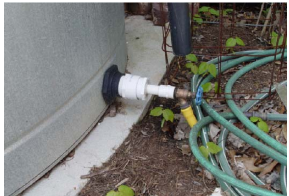
Figure 5 Bulkhead fitting installed at the base of a cistern.
