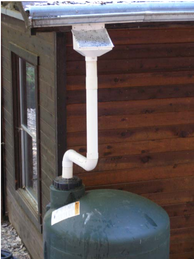
Figure 8 Rain barrel for landscape watering. Note the leaf guard over the gutter screen and strainer basket, which are used to reduce clogging and maintenance.
