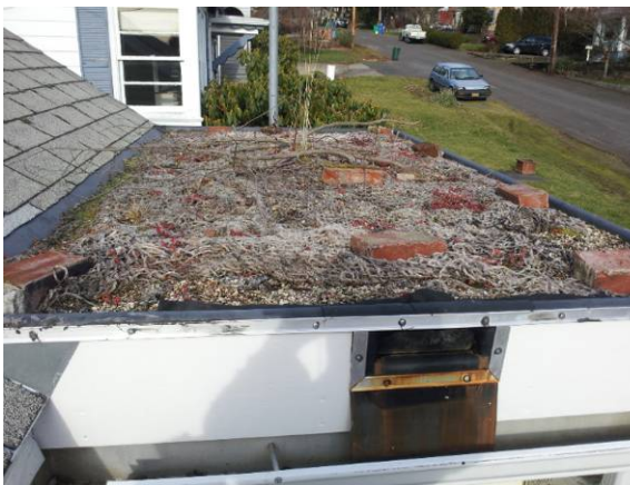
Figure 6 Ecoroofs intercept & evaporate rainfall and greatly extend roof life.
