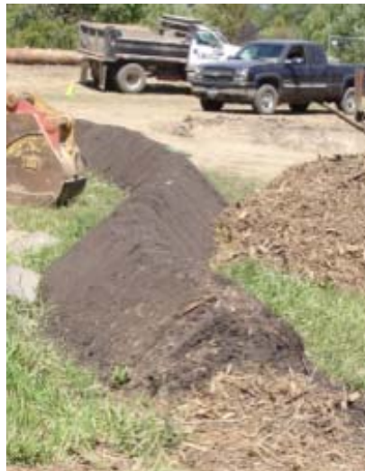
Figure 2 This berm, made of compost instead of ordinary loose soil, is highly effective at reducing sediment transport off-site and can be installed by hand or machine.
