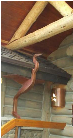
Figure 1 Choose good materials and avoid polluting ones (like this copper downspout).
