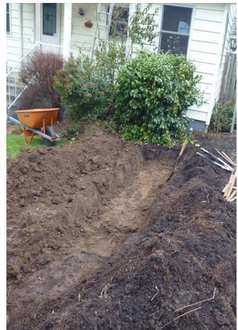
Figure 6. This vegetated conveyance swale will be partially lined, which is why it's so deep.
