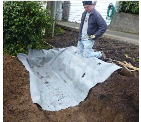
Figure 7. A single sheet of EPDM is being laid in the bottom to a minimum distance of 10' from the house.
