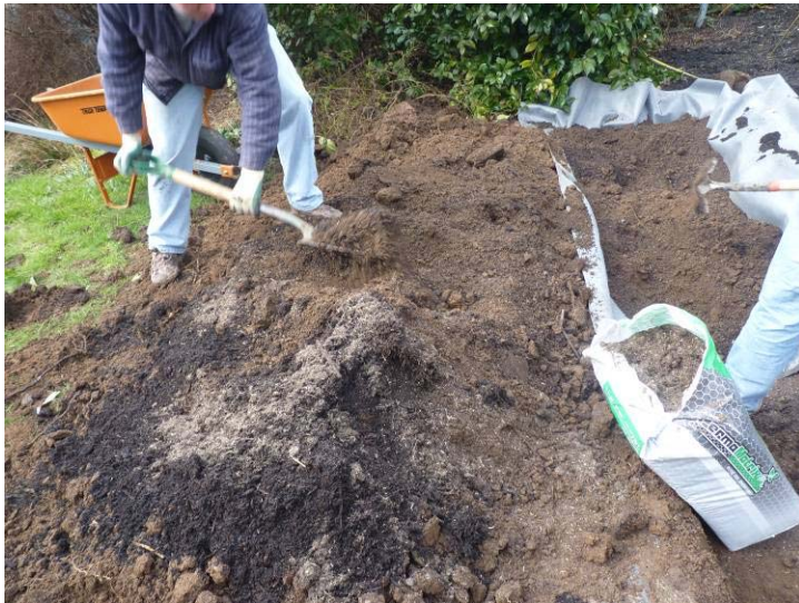
Figure 9. A few inches of compost and a sprinkling of a soil restoration product with mycorrhizae and biota (Permatatrix used here) were placed over native soils, then shoveled together and into the swale.
