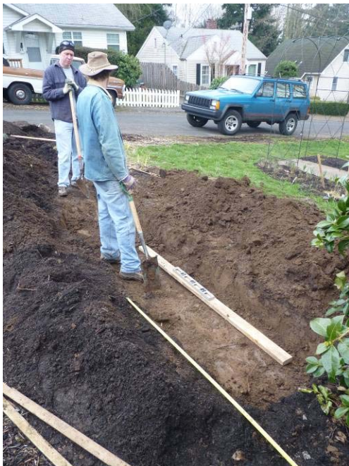
Figure 8. Since the bottom of the lined swale will empty into native soil, the bottom of the swale must also slope away from the building. Otherwise, plant roots won't dry out between waterings and rainfall events or plants won't be healthy.
