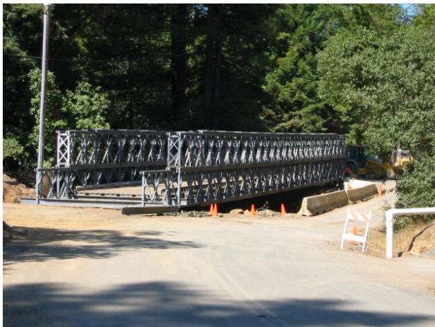
Baily Bridge detour on the Albion River.
