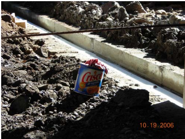
Environmentally friendly non-petroleum based lubricants so arch elements could be pushed in place under the Albion River detour.
