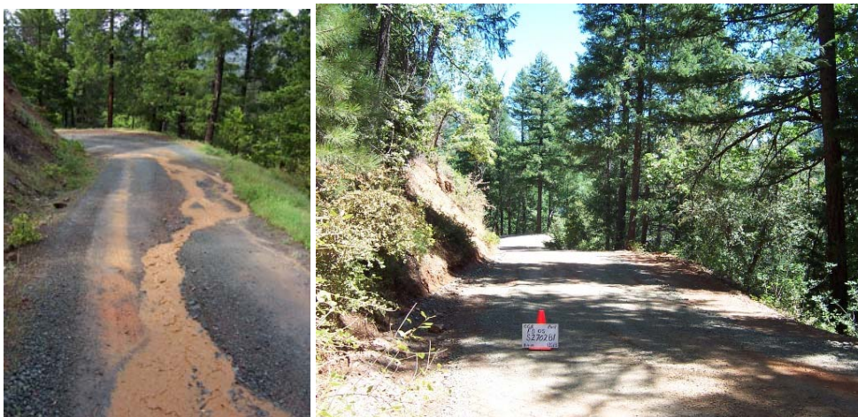
Above left pre-project ditch diversion down the road. Above right post project outcropping, ditch removal and rolling dips drain water across the road rather than down it. Below pre-project culvert misaligned and directed into bank was replaced with a proper aligned and larger culvert
