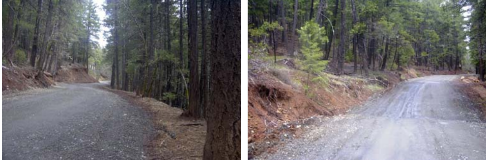
Outsloped segments of the south side of China Gulch Road repaired in 2001 reduced bank slides, ditch down cutting, road gullying and fill failures. There has been no maintenance on this road in the intervening nine years except for slide removal at Site 2464.1
