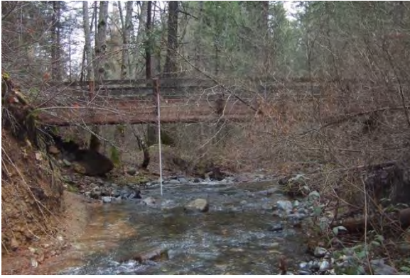
Figure 10-2: East Weaver Campground Pedestrian Bridge Spans the entire floodplain of East Weaver Creek.
