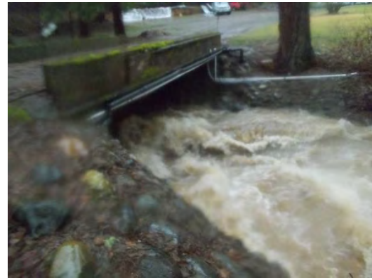
Figure 10-5: Butterfield Private Road Bridge in December 2015 (Above Left) and in January 2016 during an estimated Q2-Q4 storm flow.
