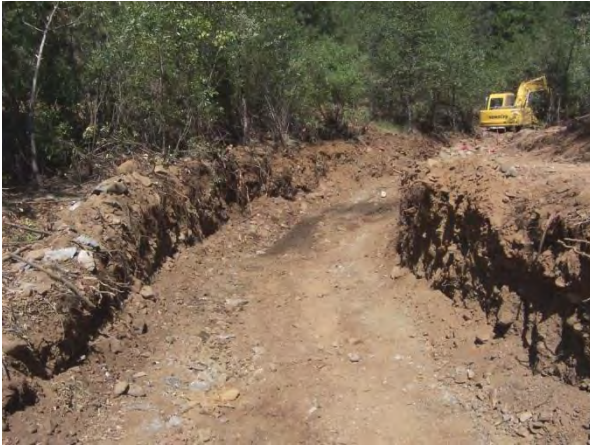
Figure 7-4: A section of Little Browns Creek dewatered, aggraded materials removed and excavation below the channel grade in order to install streambed materials and grade control structures. The excavation provided mechanical access to the stream reach.
