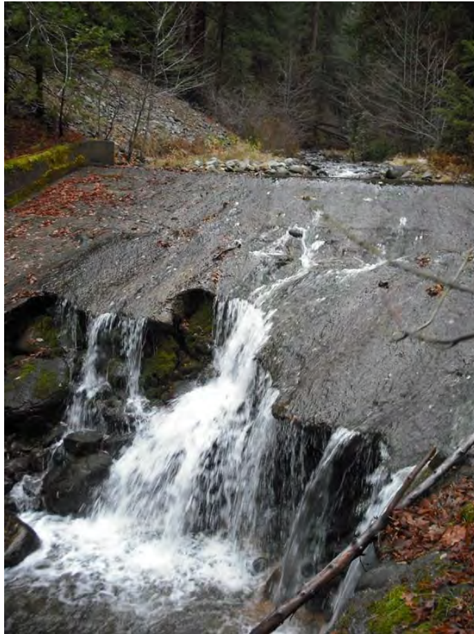
i: East Weaver Dam- integrity of the structure has been compromised by undercutting.
