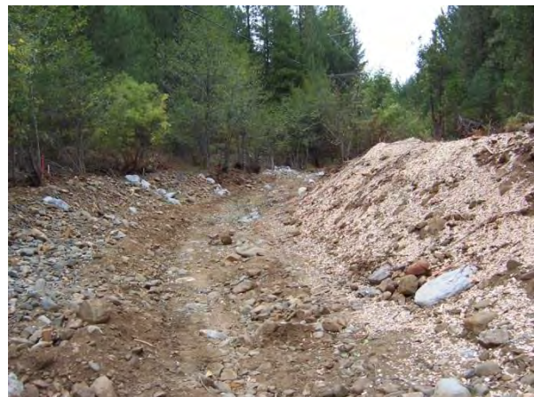
Figure 7-7: Grade control veins are buried every 25' and the channel bottom bedload materials in place (final jetting and washing fines has not been done at this stage).
