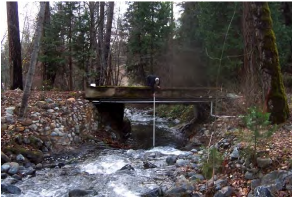
Figure 10-4: Butterfield Private Road Bridge shown in December 2015 is the most undersized crossing.
