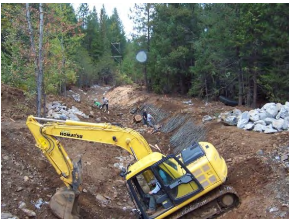
Figure 7-6: Construction of grade control veins into the banks and below channel grade (note: grade control boulders and willow plantings materials in background).
