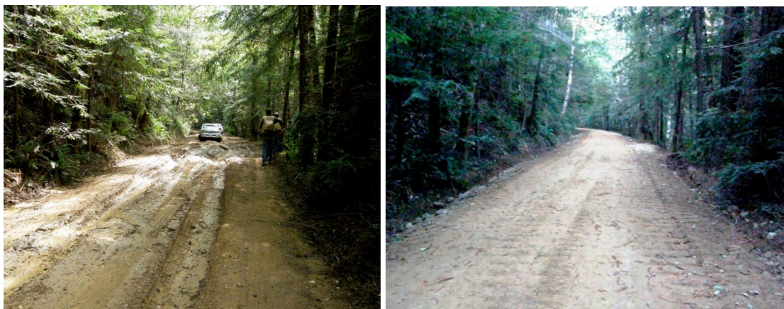
Figure 1. the lower “Quagmire” site ~400’ south of Waterfall Gulch before (left) and after (right). The treatment included outslope with berm breaks, non-woven geo-textile fabric, 8” of roller compacted rock surfacing, and upgraded stream crossings (Photos by Richard Gienger).
