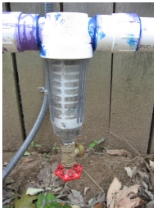
Figure 4. An inline filter can reduce sediment that will clog trickle and drip irrigation lines. The valve at the bottom allows you to drain sediment and the plastic casing screws off to give you access to the screen filter.
