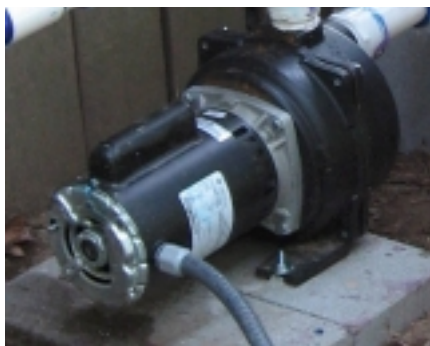
Figure 7. This 1.5 hp pump is used to irrigate shiitake mushrooms and 1/2 acre of organic vegetables using a mist system and soaker hoses.
