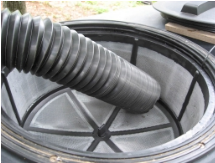
Figure 5. A screened basket in the manway hole will prevent a lot of organic matter and mosquitoes from entering the tank.
