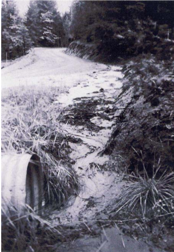
A. Before – Insloped, unsurfaced road on decomposed granitic soils with heavy sediment runoff
